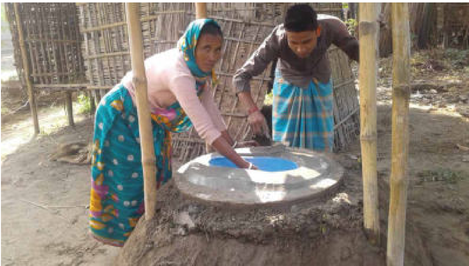
Photo 44: Participants building toilet for better sanitation through support from SWARP (ESDO-Water Aid Bangladesh)
